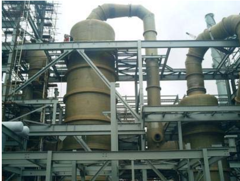
Figure 5. Gas cooling tower and final DynaWave® scrubber for a spent acid regeneration plant under construction
