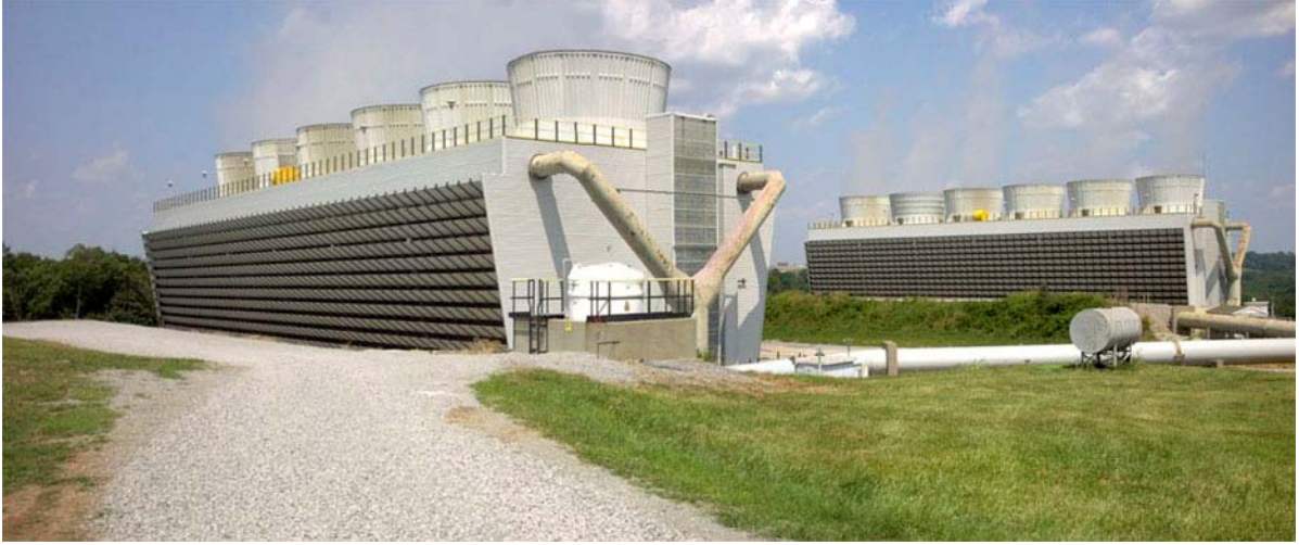
Figure 18. All FRP Cooling Towers
