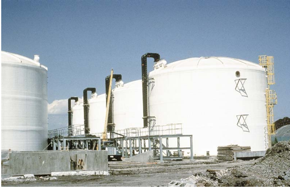
Figure 14. Large Field Wound Hot Water Storage Tanks
