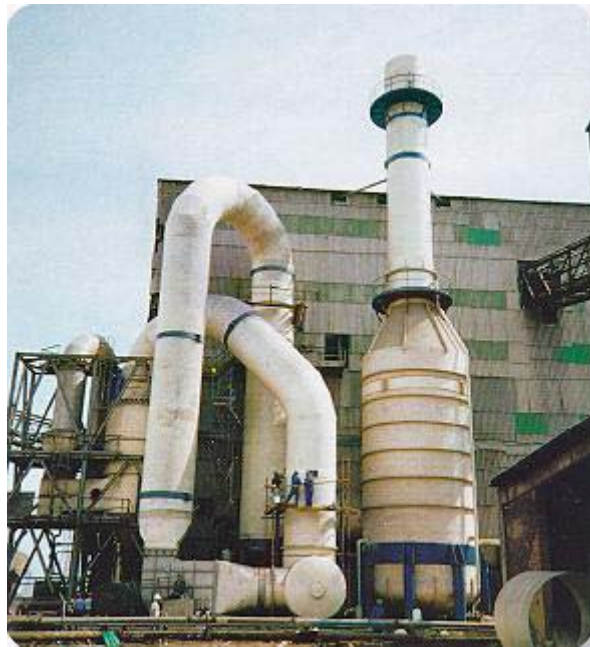
Figure 4. Scrubber in Diammonium Phosphate Process
